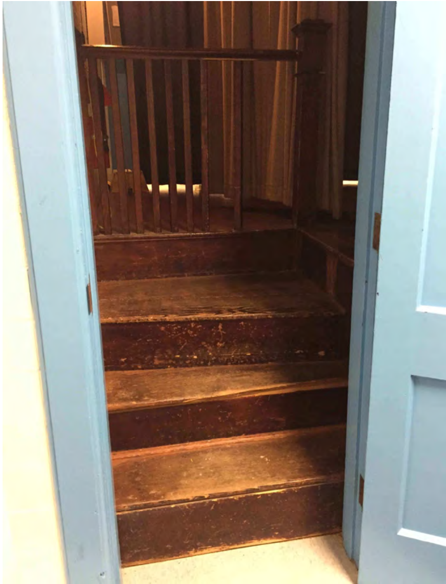
Stage stair is not Handicap accessible
